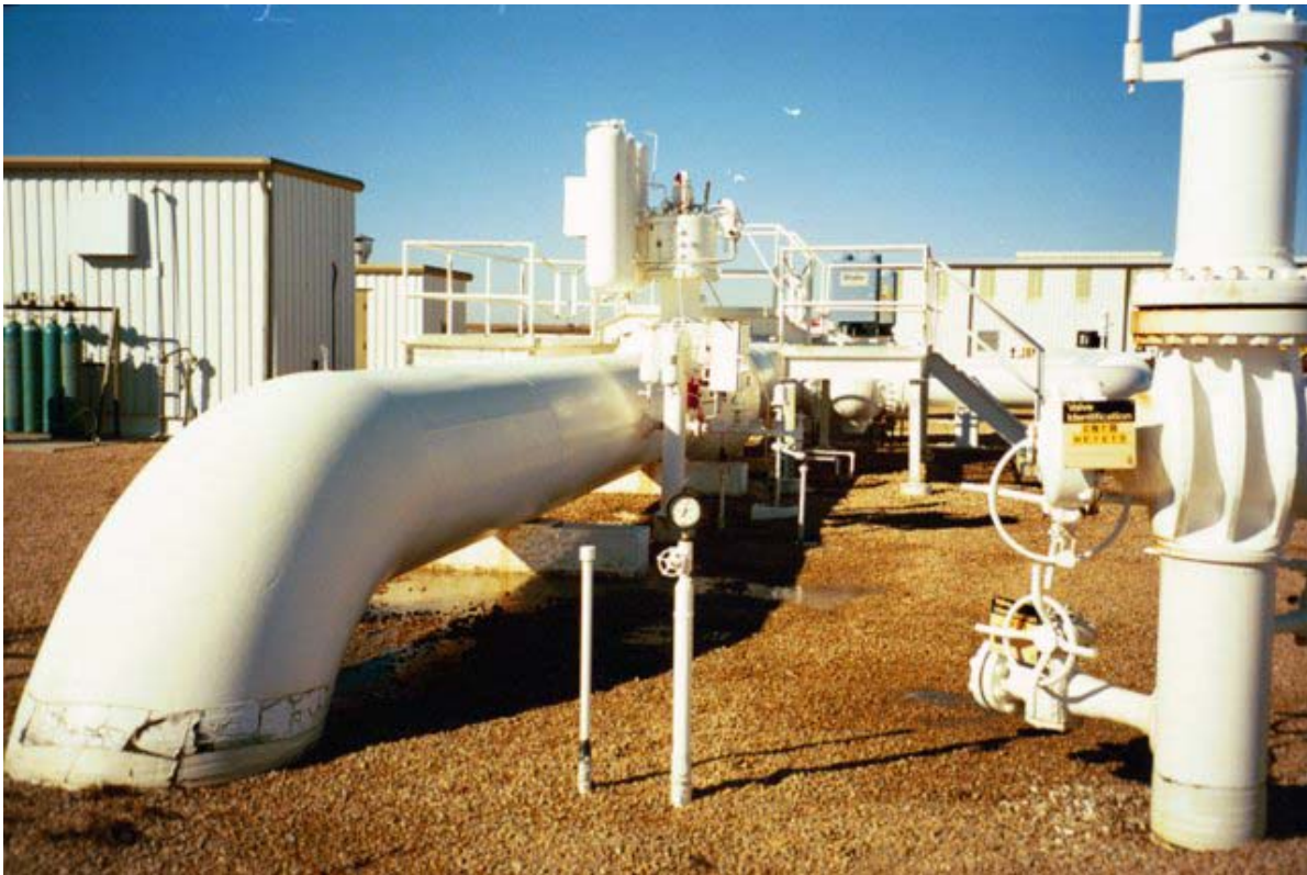
CEESI flow calibration facility, Garner, Iowa Photo by Flow Research
